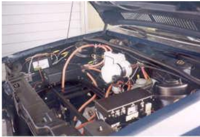
Low and high voltage wiring of the components
